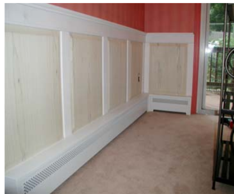
#6 – Radiant Wraps slipped into place and installation complete. Wainscoting to be painted.
