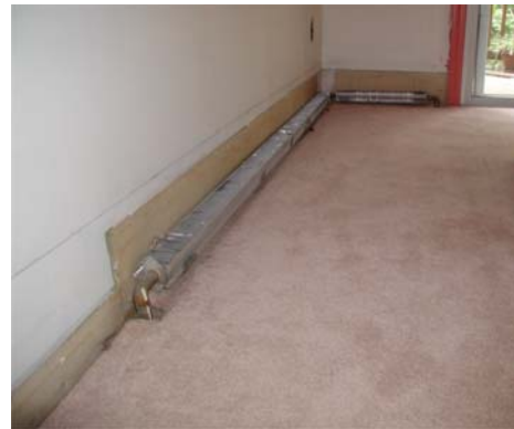
#2 – Baseboard enclosure removed prior to wainscoting layout and installation. Refer to Removing Back Panel .
