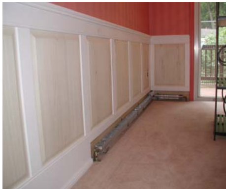
#3 – Unfinished wainscoting installed. Location and height of base molding determined by Radiant Wraps.
