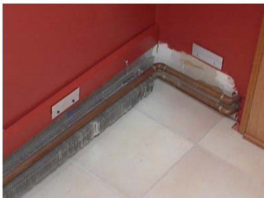
#5 – Install mounting brackets to spacer board at the appropriate height off the floor.
