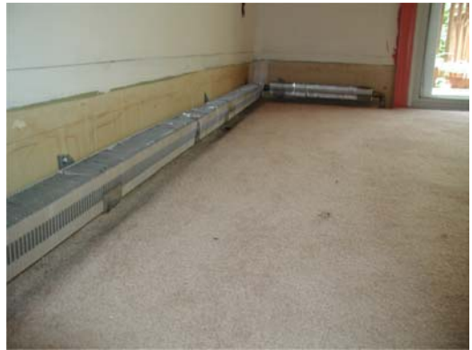
#6 – This photo shows the heating element and support brackets re-installed after removal of the back panel.
