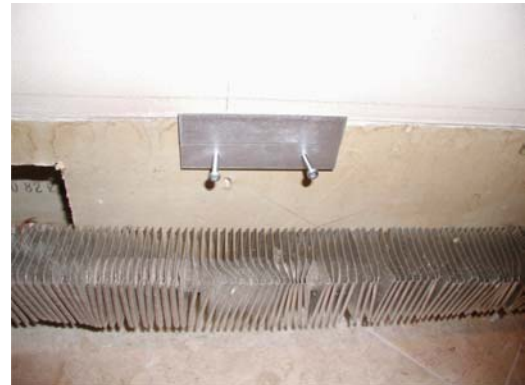
#4 – Install mounting brackets. You may have to use a small pry bar to widen the gap off the wall at the top of the bracket.
