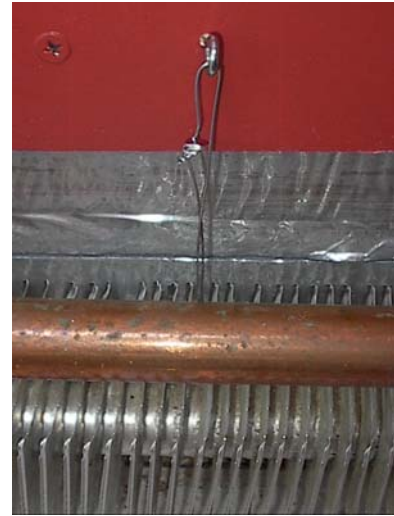
#2 – Close up view of eye-hook installation and wire support of heating element.
