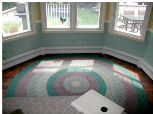
#4 – This picture shows the finished bay window with multiple top rail wedge pieces.
