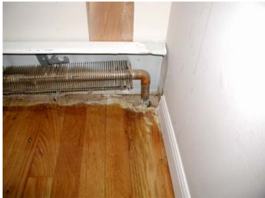
#1 – Back panel extends in to or is flush against an intersecting wall. Use shim to create space off the back wall.
