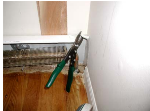
#2 – Use metal snips to slice top rail first. Be careful of sharp edges.
