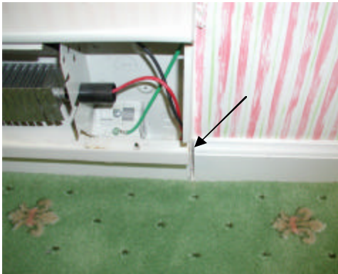
#3 – Note the notch that is being cut into the wooden base molding to allow the new Radiant Wraps end cap to slip down along the wall and rest firmly on the floor.
