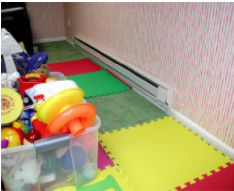
#1 – Note that the electric baseboard heating unit has been installed in an elevated position above the wooden base molding. This is not unusual.
