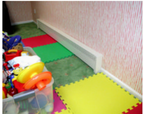
#4 – Photo of the new Radiant Wraps section that has been slipped on over the existing electric unit.
