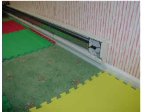
#2 – The electric baseboard heating unit with all snap-on face panels and covers removed in preparation for the Radiant Wraps retrofit.
