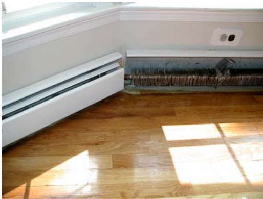
#1 – The retrofit of a non-90 degree corner requires the use of a Radiant Wraps' measuring gauge to determine the final length of each intersecting panel.
