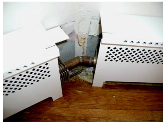
#2 – The positioning of the two intersecting panels (determined by the measuring gauge) will allow for the left and right open end caps to create the new corner.
